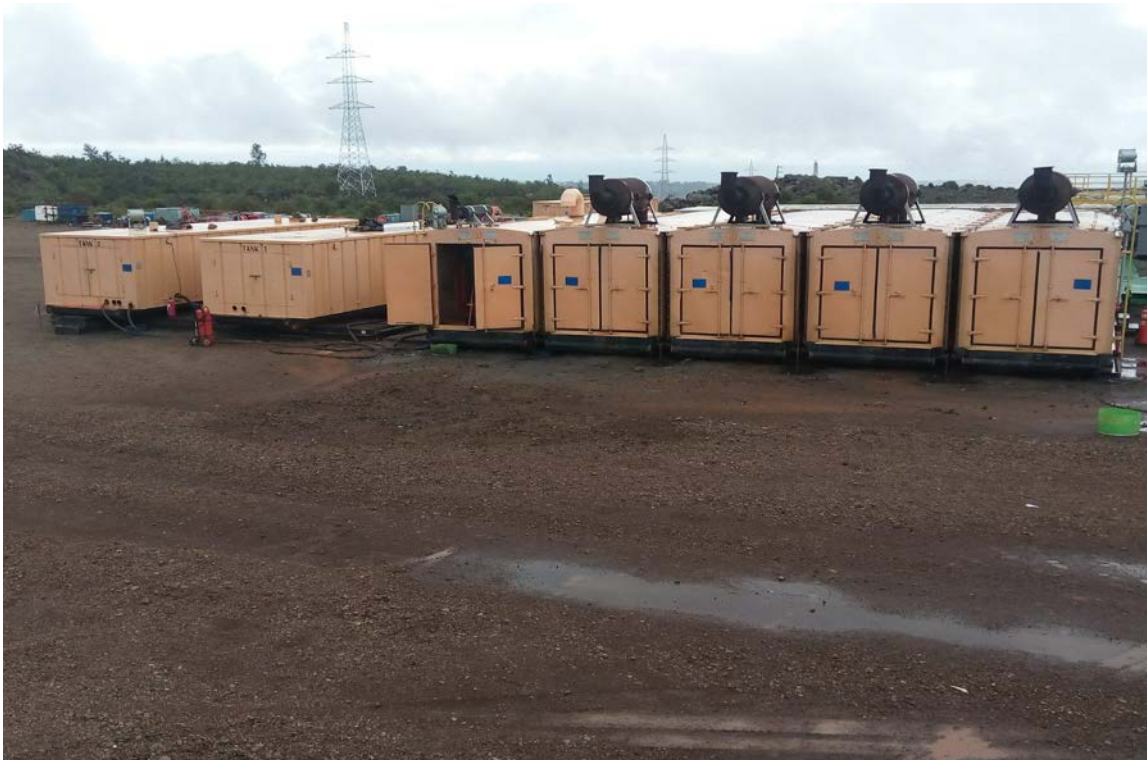
FIGURE 1: Diesel tanks and power generating unit
