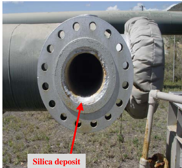
FIGURE 3: Silica scale forming in a steam delivery line (Photo courtesy James Wambugu)
