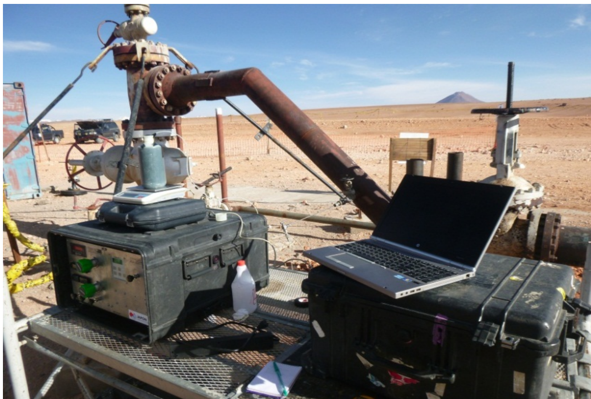
FIGURE 1: Installation of MicroMod Tracer Injection Unit (TFT method) during well testing of SM – 03 in February 2013
