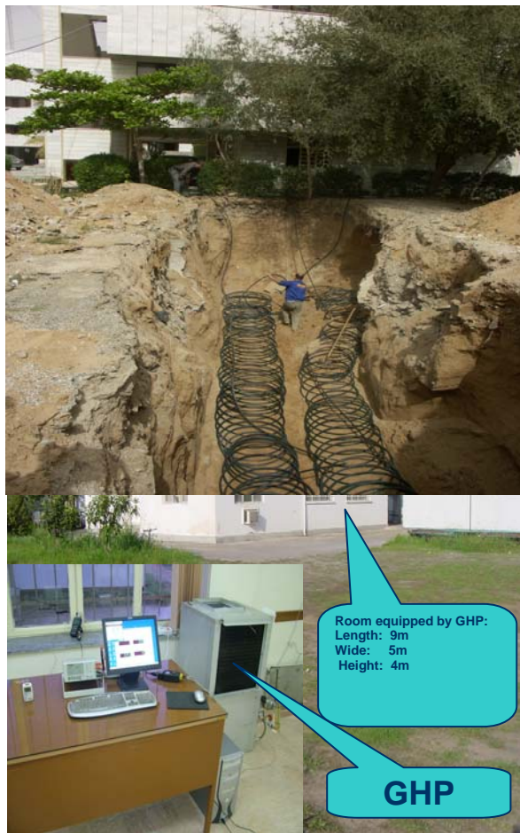
Figure 5. GHP with slink loop installed in 2007 (Bandar-Abbas)
