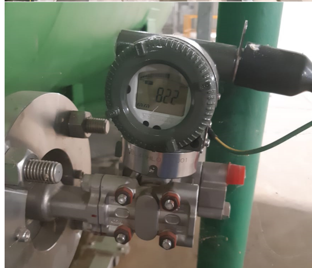
FIGURE 7: Field instruments in Ulubelu units 3 and 4 used for monitoring and control
