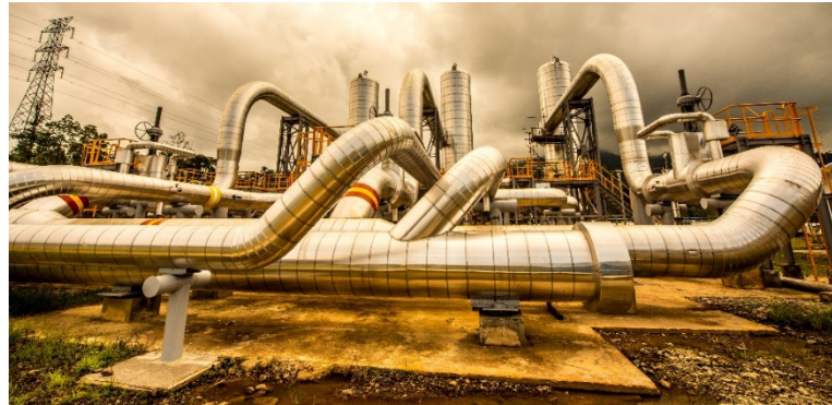
FIGURE 3: The centralized separator in the Ulubelu units 3 and 4
