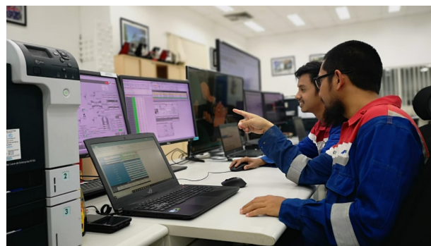
FIGURE 8: Operators operating power plant in control room for Ulubelu units 3 and 4
