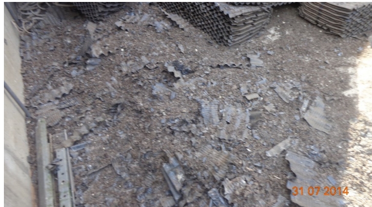
FIGURE 16: Debris that had accumulated in the cooling tower film fills before the major overhaul
