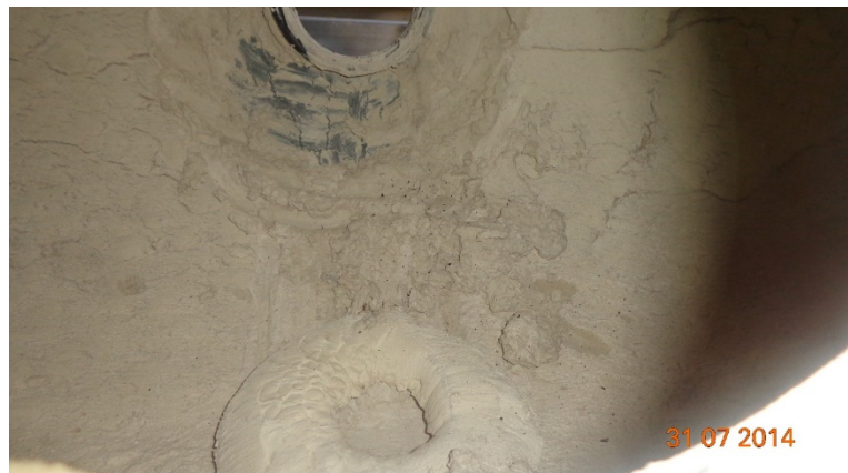
FIGURE 17: Accumulated sulphur deposits in the common header of the distribution pipes
