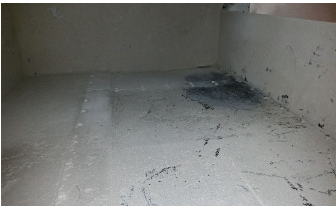
FIGURE 11: Gas cooler trays clogged by elemental sulphur
