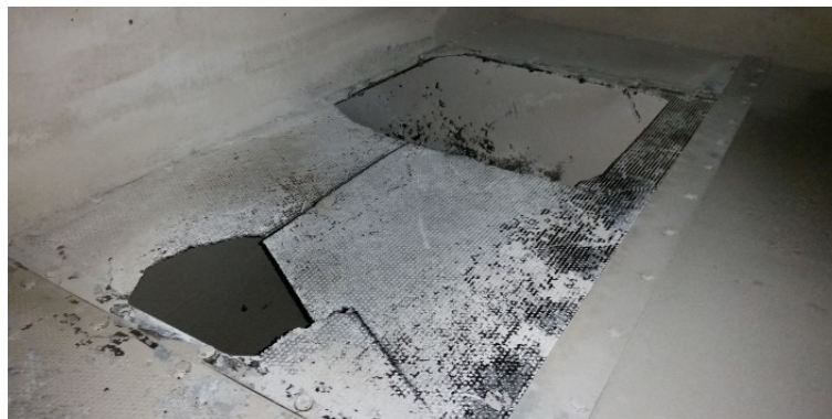
FIGURE 12: Gas cooler trays broken due to the weight of accumulated cooling water
