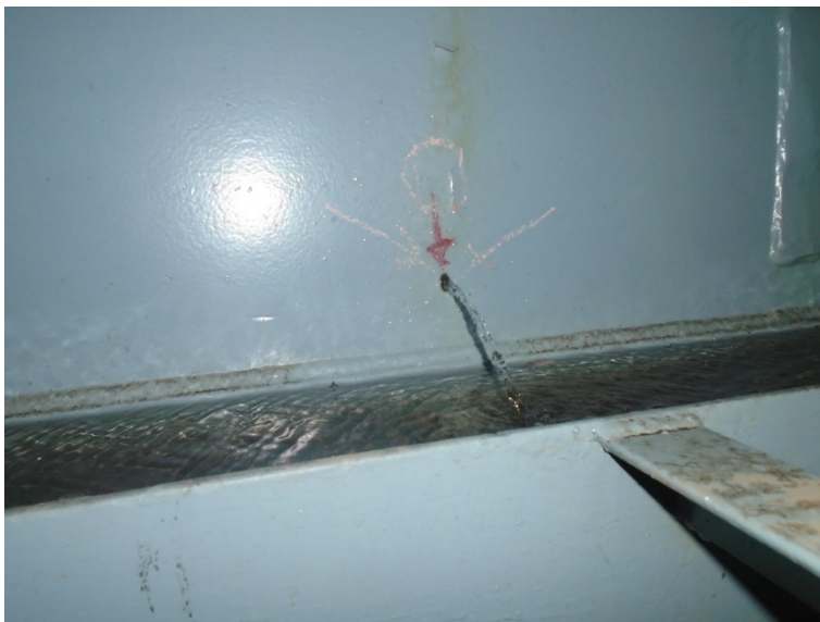
FIGURE 23: A jet of water flowing out of a hole in the unit 2 condenser shell in 2018 at the top of the cooling tower
