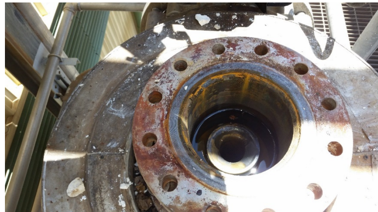
FIGURE 18: Ejector opened during annual inspection in 2016
