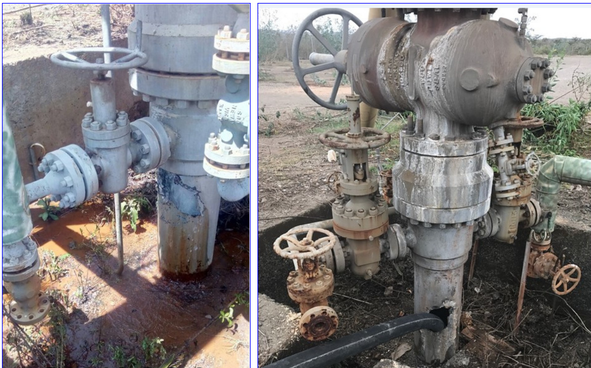
FIGURE 3: Corrosion in condensate disposal wells in Olkaria field (KenGen, 2017)
