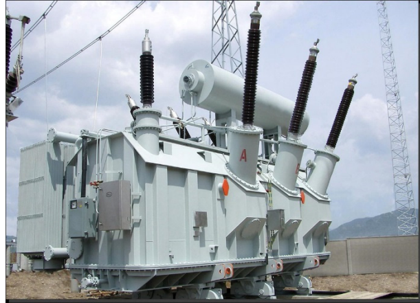
FIGURE 4: A power transformer
