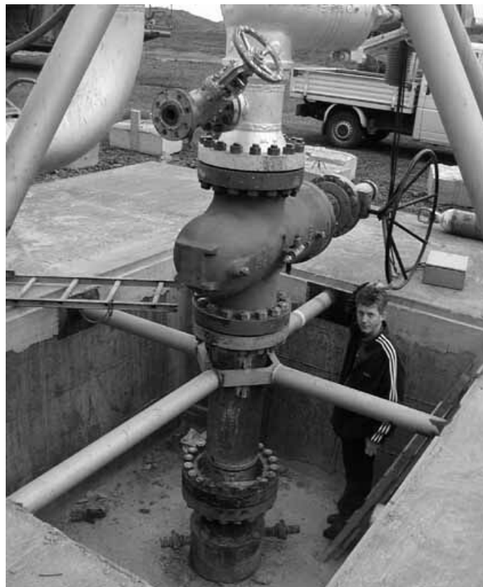
Figure 2: Wellhead with a locally fabricated expansion spool, without annulus pressure seal or side outlets below the master valve. Side outlet above master valve is for killing.
