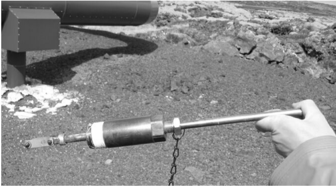
Figure 5: In-line monitoring of scaling and corrosion by use of retractable coupons.
