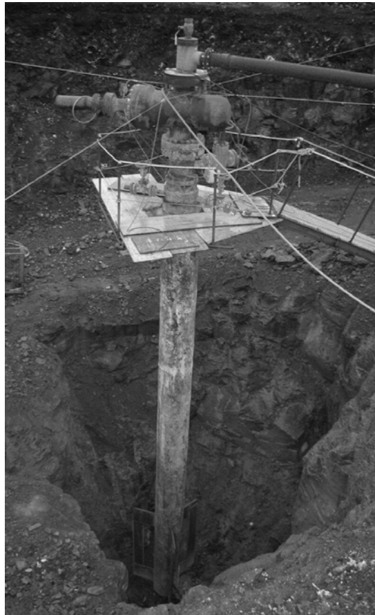
Figure 15: A hole excavated 12 m to the first casing joint where there was a leak. The top-most casing was then replaced.
