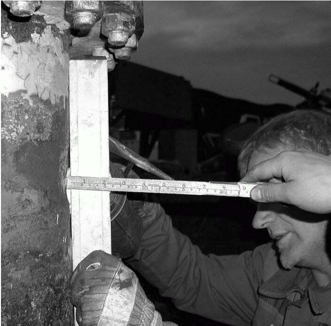
Figure 17: Corrosion on the outside of 9-5/8" casing (7 mm) at the top of cement after 20 years. Repaired with an outside patch of 10-3/4" casing and welding.
