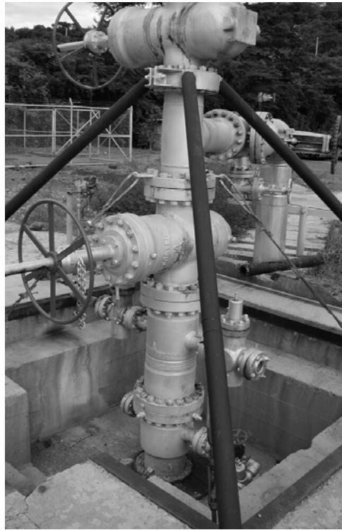
Figure 3: Wellhead with an expansion spool and pressure seal for annulus. Four side outlets.
