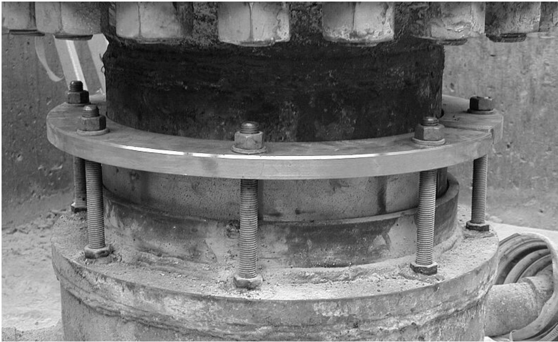
Figure 19: A gland installed on an old well to seal a leak in the annulus by the anchor casing.
