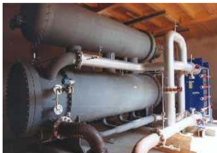
Figure 25: Power plant building and evaporator/condenser of the ORC-circuit in Altheim (photo: O. Joswig).
