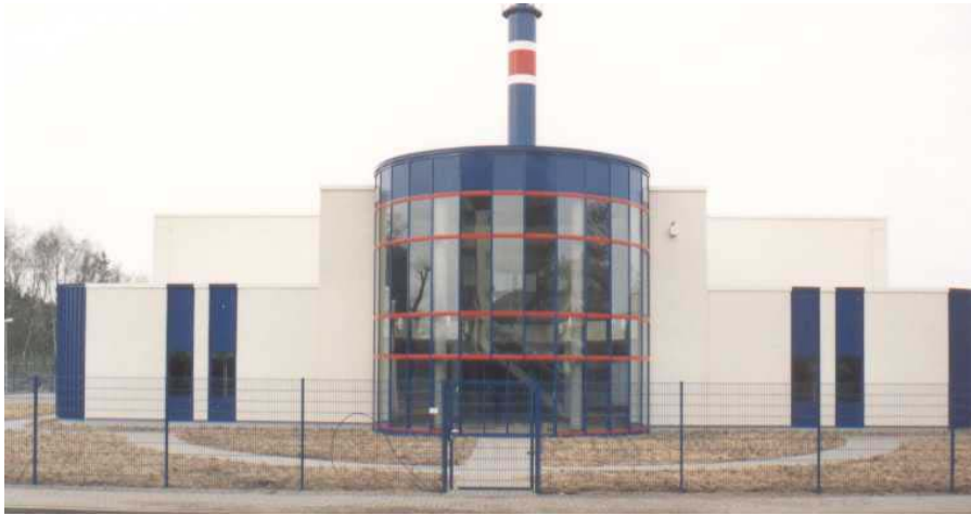
Figure 26: Geothermal district heating plant Neustadt-Glewe, central building with control, heat exchangers, district heating circuit pumps and peak boilers (photo: O. Joswig).
