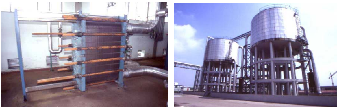
Figure 5: Ferrara geothermal district heating, Italy. Left: Plate heat exchanger. Right: Hot-water storage tanks beside the waste incineration station (photos: O. Joswig).
