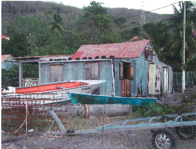
Photo 3. A house near the pipeline where the floor is hot and deposits on the outside of the foundations. The stone stairs to the main door under the window issue steam at 98,9°C.
